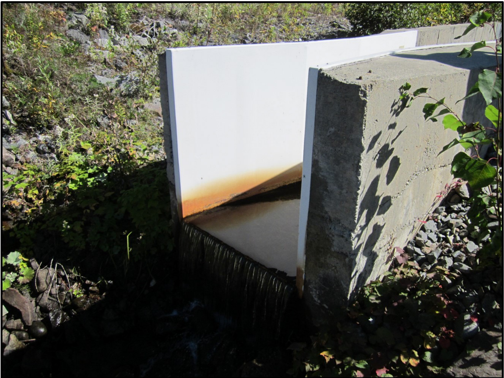
Photograph 4: Final effluent point
